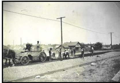
Washington Paving Co. crew paving Commercial Avenue for the first time in 1914. Photo is taken at 26 th Street looking west.
